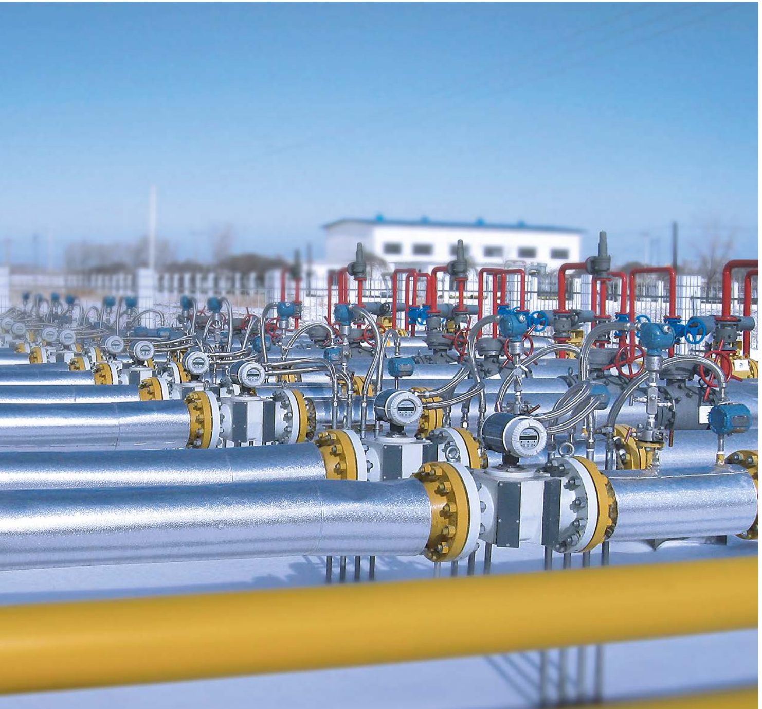
Natural gas pipeline in Bawu-Changnan using FLOWSIC600
