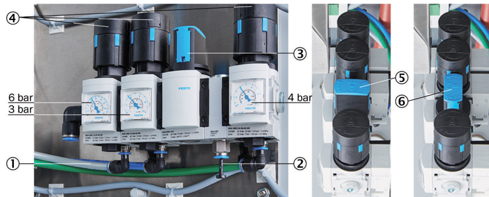
Figure 54: Pressure reducer unit
