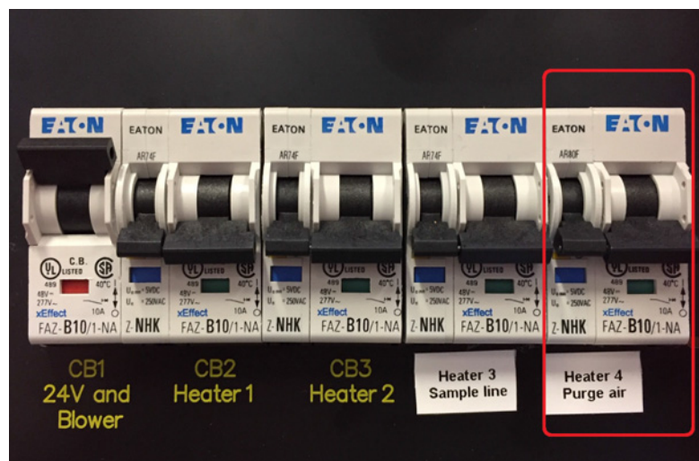
Fig. 14: CB5 fuse for the purge air heater
