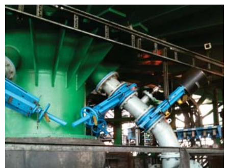
Coal Washing Plant
